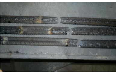
Failure sections in G3
